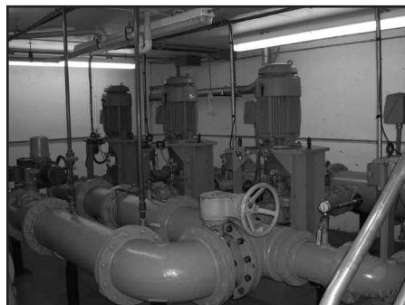
Pumping stations help City operators distribute water to meet fluctuating daily consumption requirements.
