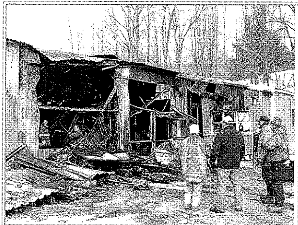
Investigators survey the fire damage at the Ashland Town Hall and Fire Department Sunday afternoon. (Mike Ryan/Hudson-Catskill Newspapers)
